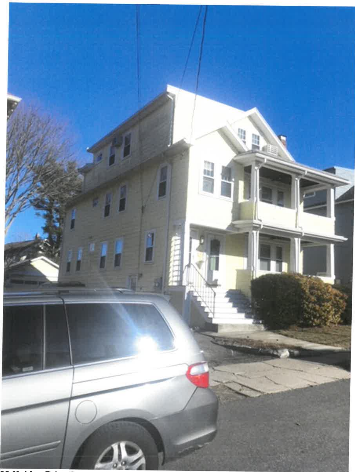
23 Holden Rd. – Dormer. Large portion of foundation is exposed.
