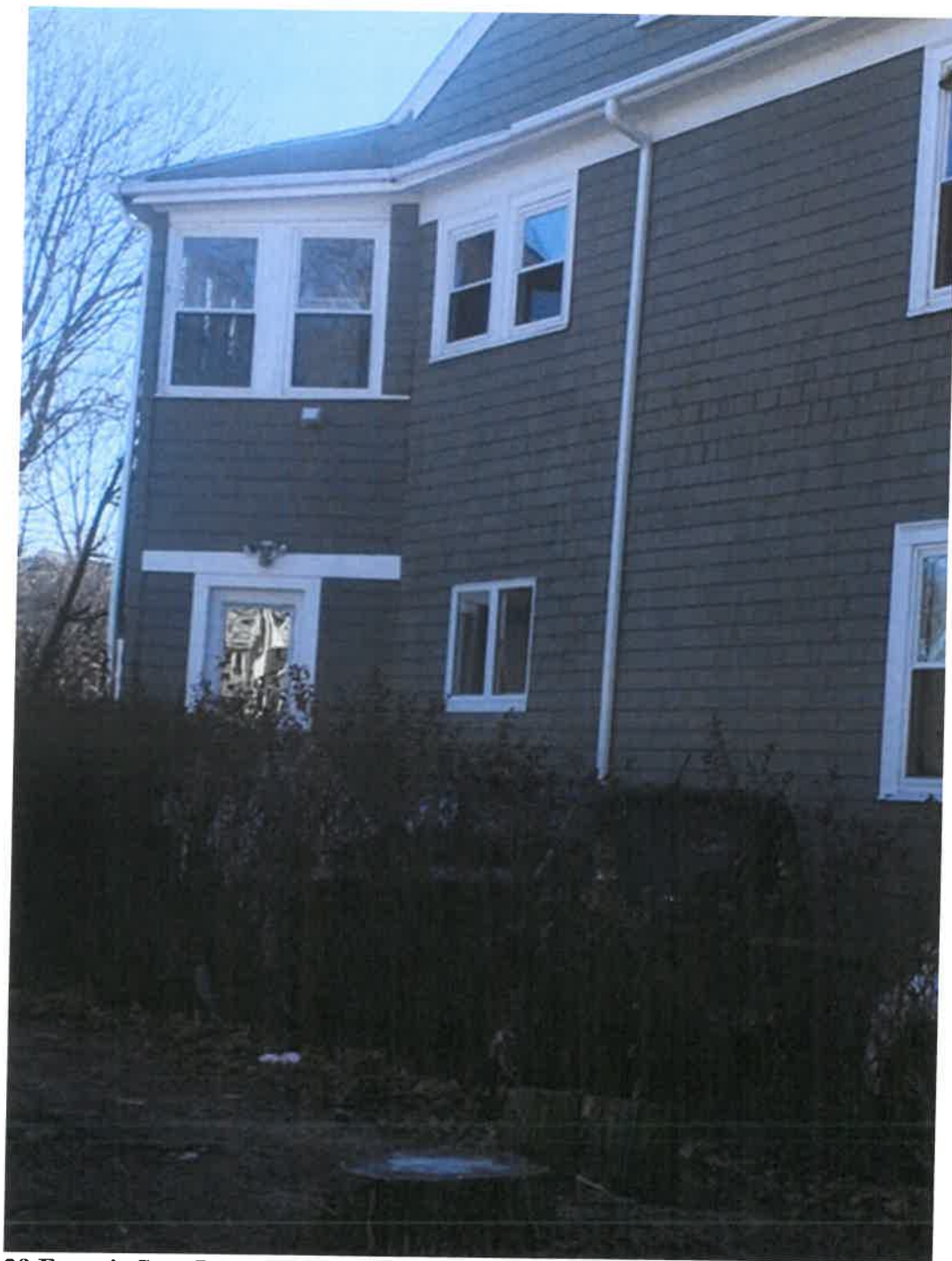
29 Francis St. – Rear porch enclosed, both stories. We are only proposing to enclose a portion of first story rear porch.
