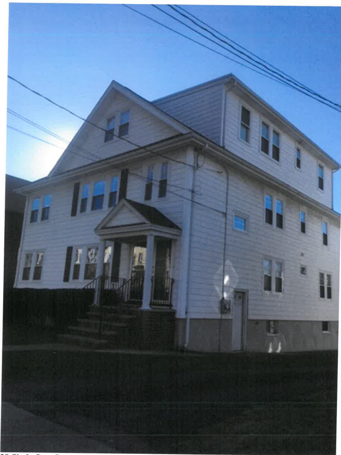
38 Slade St. – Dormer. Large portion of foundation exposed.
