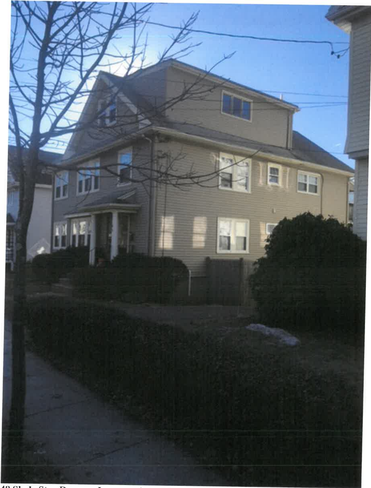
48 Slade St. – Dormer. Large portion of foundation is exposed.
