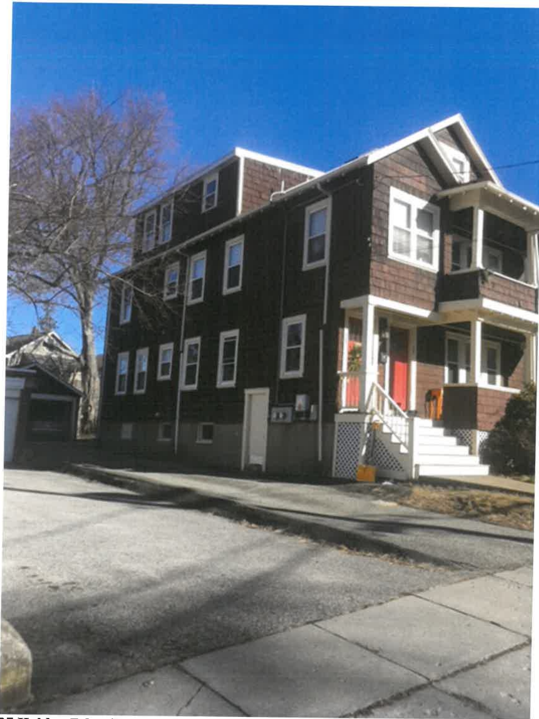
27 Holden Rd. – Dormer. Large portion of foundation is exposed.
