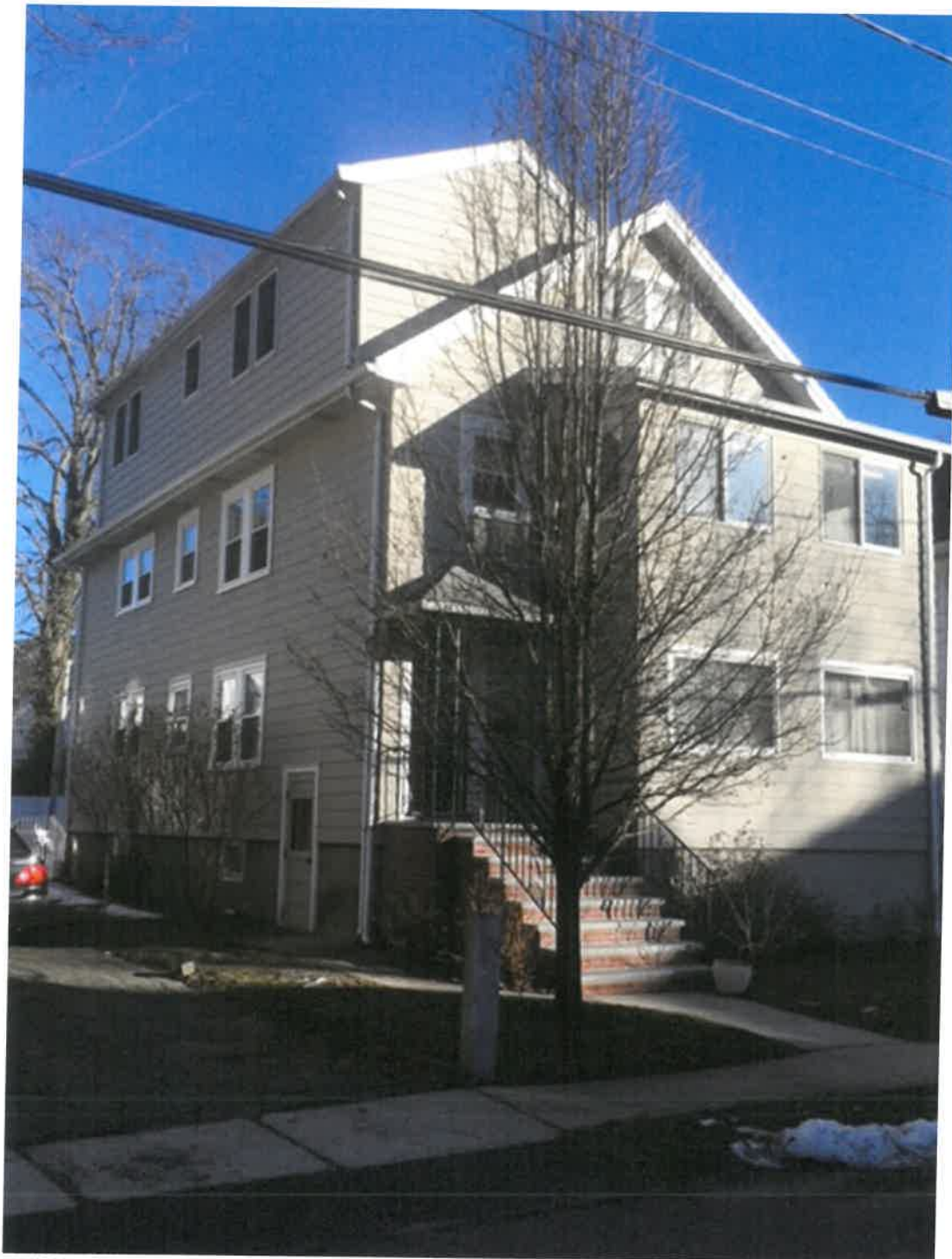
49 Flett Rd. – Dormer that extends above ridge of existing house. Large amount of exposed foundation. Two-story enclosed front porch.
