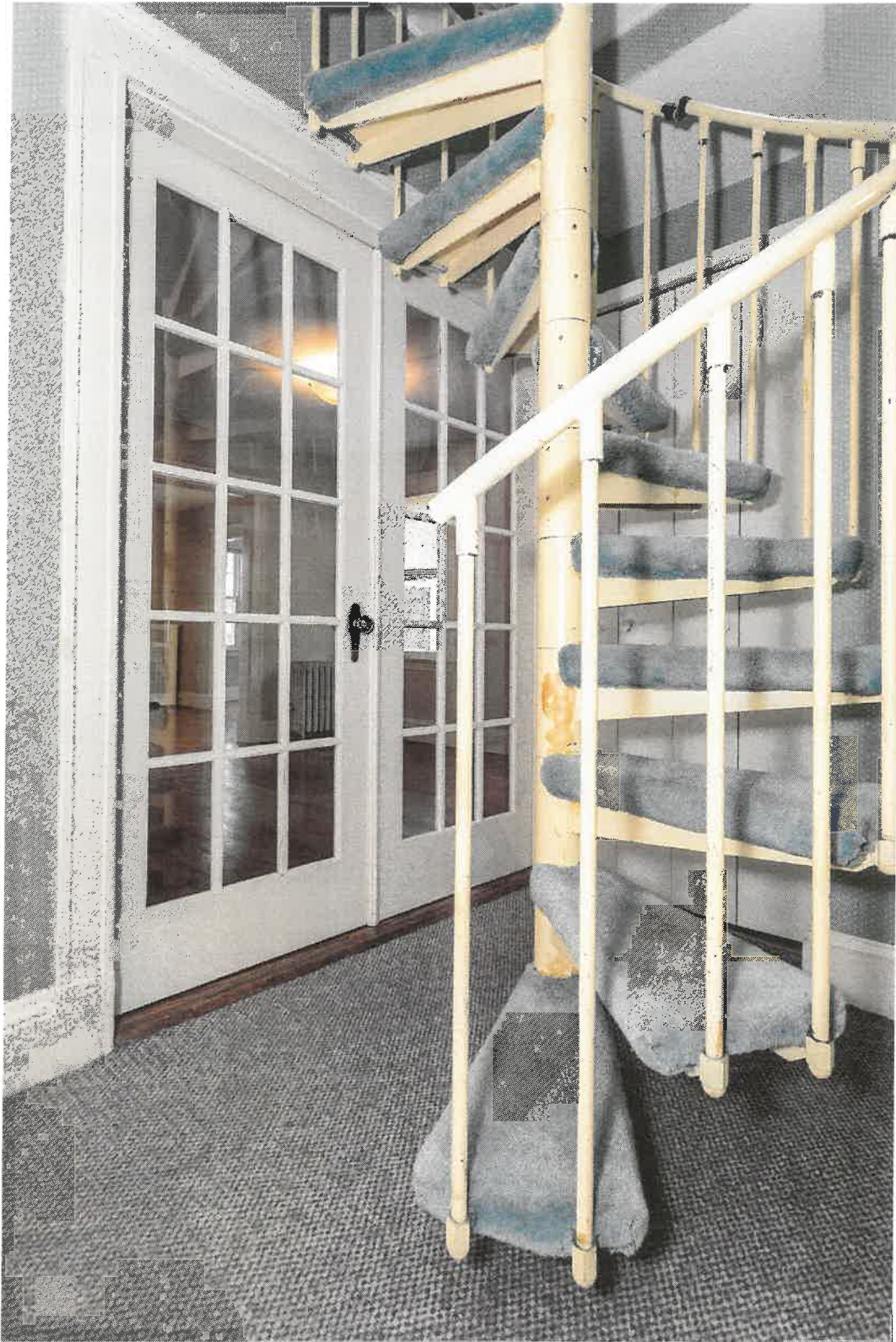
Picture F – Non-conforming spiral stair – main level
